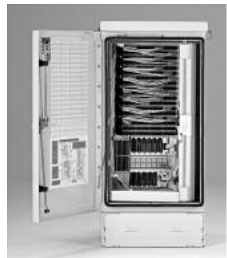
OptiTect Premier Cabinet - Open (432 fibers) | Photo HWPSS1752
